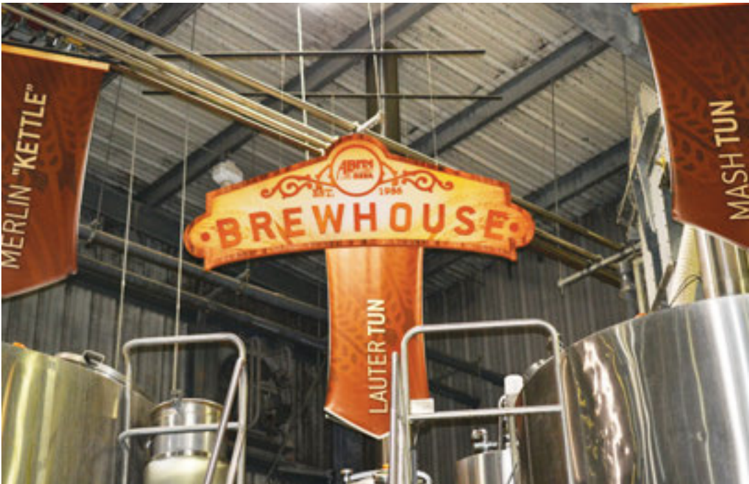
The new 200-barrel brewhouse installed by Krones that came on line this spring is part of a $12 million expansion that includes the visitor center and offices. The brewhouse features the Steinecker EquiTherm system for energy recovery.
